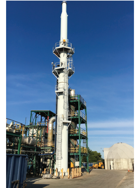
Lubrizol Painesville Waste Heat Recovery Incinerator
