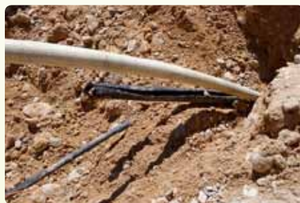
Using a splitter, a 1" FlowGuard Bendable composite pipe is easily pulled through 3/4" buried pipe in a replacement job.
