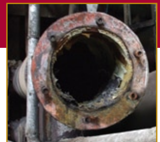
Metal pipe shown here exhibiting both internal and external corrosion.
