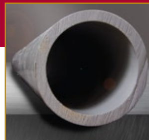
After years of service, the Corzan® pipe shows no sign of corrosion, scaling or degradation.
