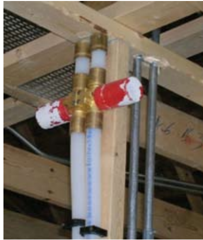
A PEX multipurpose residential fire sprinkler system used in a sidewall sprinkler head installation. (Photo courtesy of Lubrizol Corp.)
