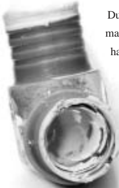
This polybutylene pipe looks fine on the outside despite the internal decay and flaking.
